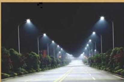
LED Street Lights
